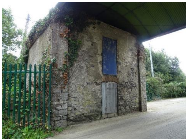
Fig.42: Coach House, east section, east elevation, vegetation overgrowth, lime render has fallen in some areas, open joint at the bottom section.
