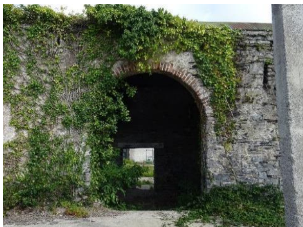
Fig.53: Coach House, West section, external south elevation, central opening, arch is leaning.
