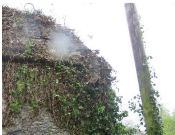
Fig.28: Coach House, east section, east elevation. Damaged gutter and cast iron rainwater pipe at the north corner.
