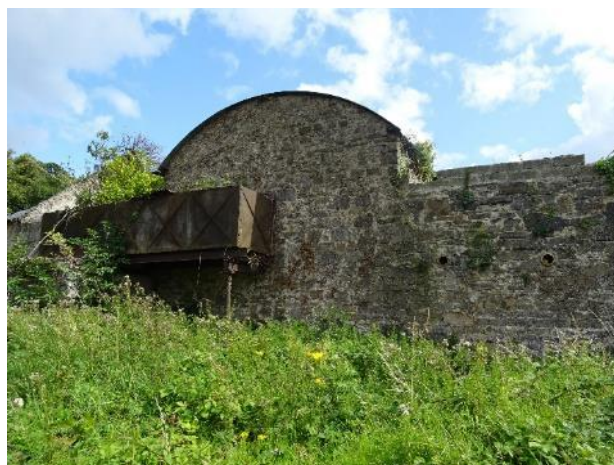
Fig.41: Coach House, west section, west elevation, the lime render has fallen.
