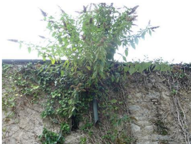
Fig.26: Coach House, west section, north elevation, section above the central door opening. Broken steel rainwater pipe and buddleia is growing.
