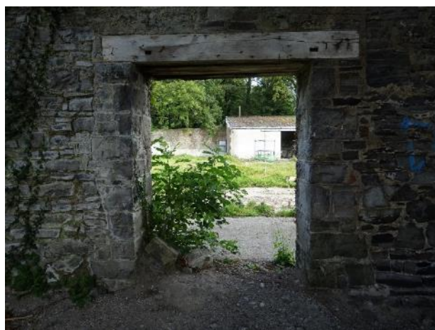
Fig.48: Coach House, West section, internal north elevation, central opening, timber lintel has cracks
