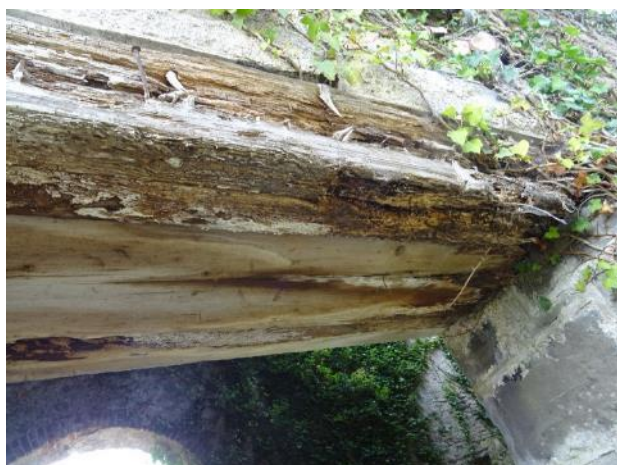
Fig.47: Coach House, West section, external north elevation, central opening, the rotten timber lintel is moving downward
