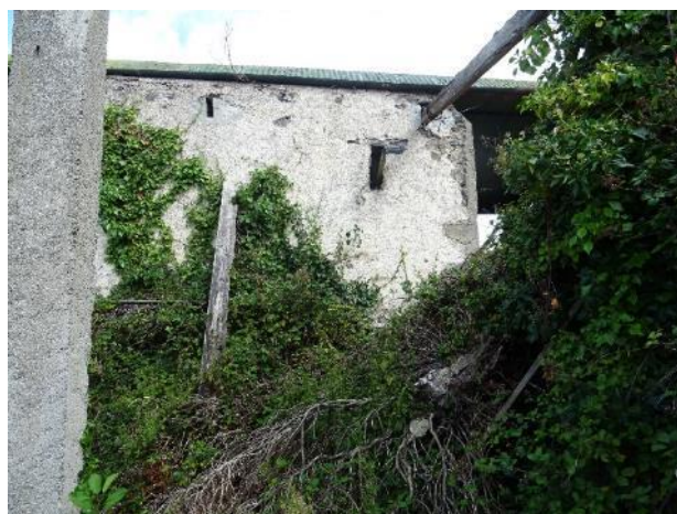
Fig.39: Coach House, west section, south elevation, concrete was cast in situ at the corner, vegetation overgrowth.
