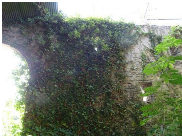
Fig.68: Coach House, west section, south internal elevation, ivy developing.
