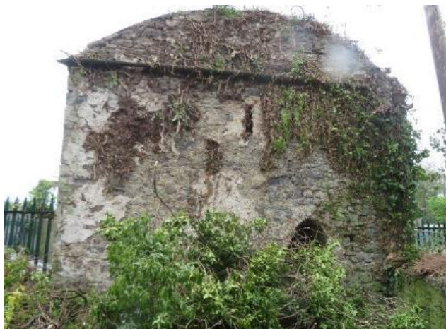
Fig.30: Coach House, east section, east elevation. Vegetation overgrowth, open joints and missing lime render.
