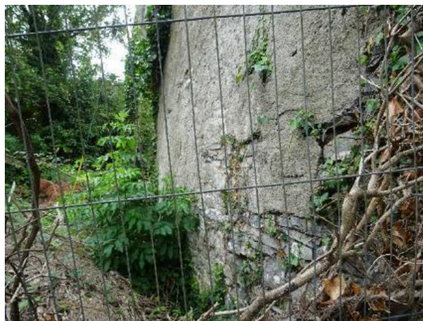
Fig.31: Coach House, east section, north elevation. Missing pointing and crack.
