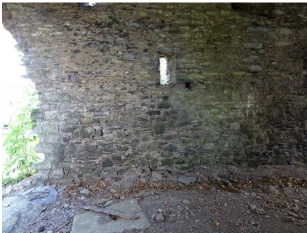
Fig.60: Coach House, west section, north internal elevation, missing stone, open joints, green moss.
