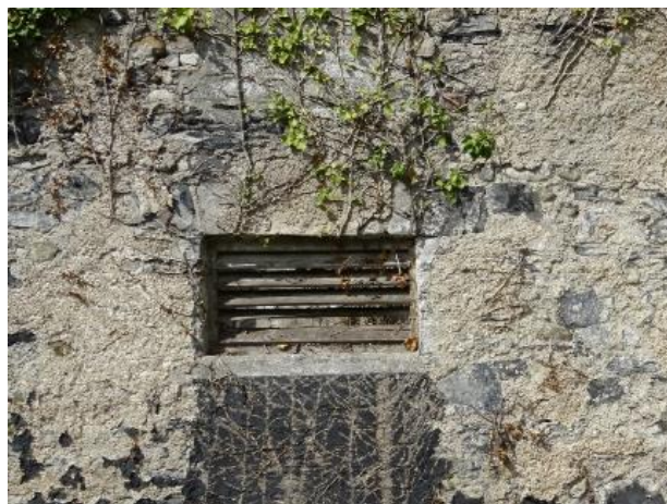
Fig.9: Barn, east external elevation, square-headed window opening were altered as there are a brick infill underneath a concrete sill.
