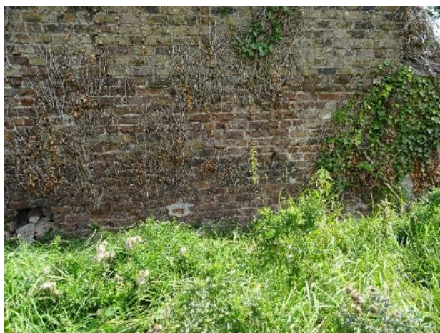
Fig.92: East wall of Walled Garden, missing brickwork to the top section, brick fair to poor condition
