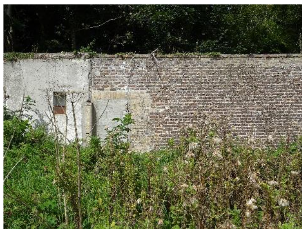
Fig.93: North wall of Walled Garden, south elevation, concrete based lime render and door opening has been boarded up with concrete blocks
