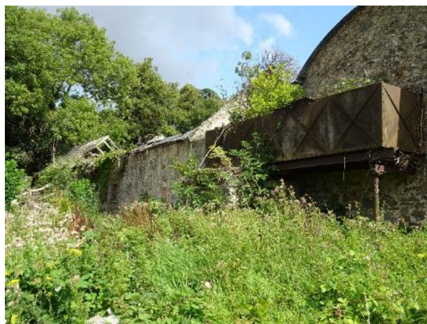
Fig.6: Barn, west elevation, lime render has fallen, vegetation overgrowth
