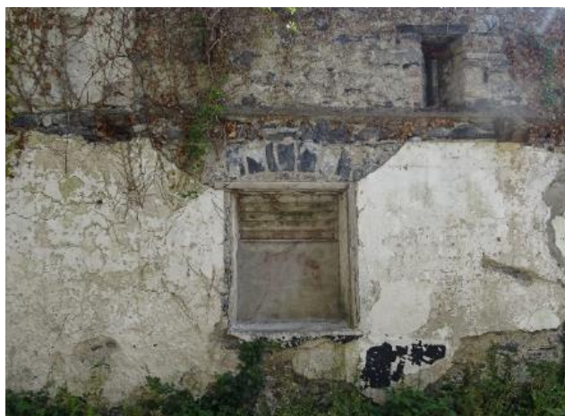
Fig.10: Barn, east internal elevation, arrow slit window at the top part was blocked-up, window opening bottom section was blocked-up.
