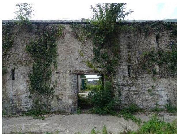
Fig.29: Coach House, west section, north elevation. Damaged steel gutter running along the elevation.
