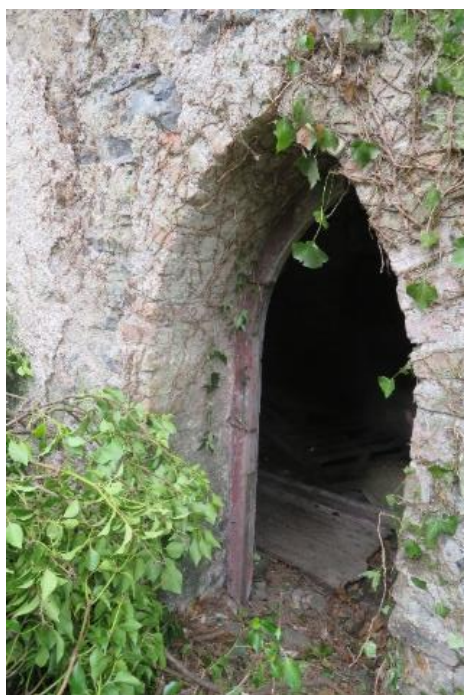
Fig.22: Coach House, east section, gothic arch door opening on the east elevation.
