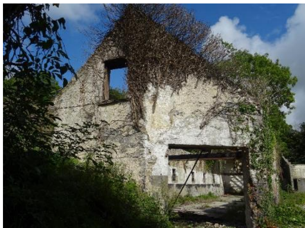
Fig.7: Barn, south elevation, lime render has degraded, vegetation overgrowth.
