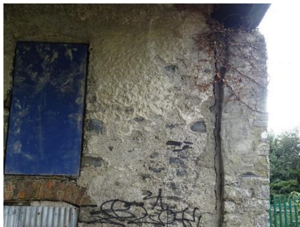
Fig.43: Coach House, east section, east elevation, crack and graffiti.
