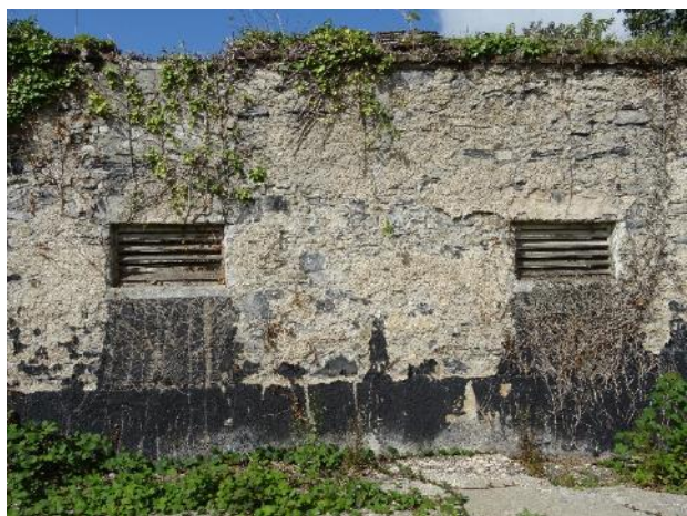
Fig.5: Barn, east elevation, bituminous paint at the bottom part, concrete brick infill below the window opening, ivy developing and lime render has fallen in some areas
