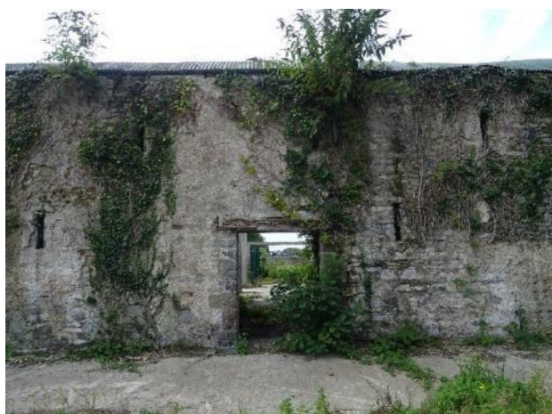
Fig.34: Coach House, west section, north elevation, remaining lime render, vegetation overgrowth.
