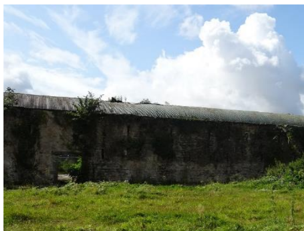
Fig.24: Looking north elevation, the corrugated metal sheeting is detaching.
