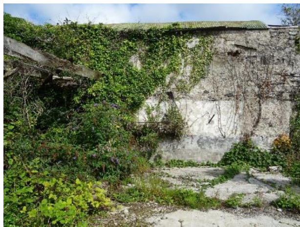
Fig.37: Coach House, west section, south elevation, cementitious render, vegetation overgrowth.
